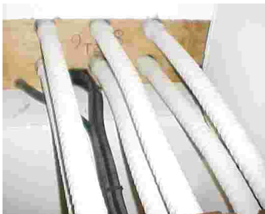
Asbestos Cable Tape in Substation
