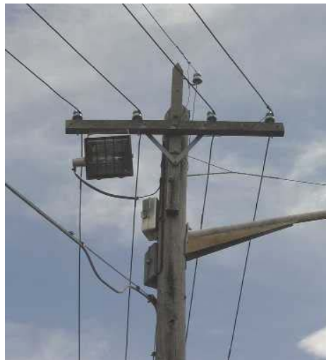
Figure 9: Single spot light mounted directly on LV cross arm
