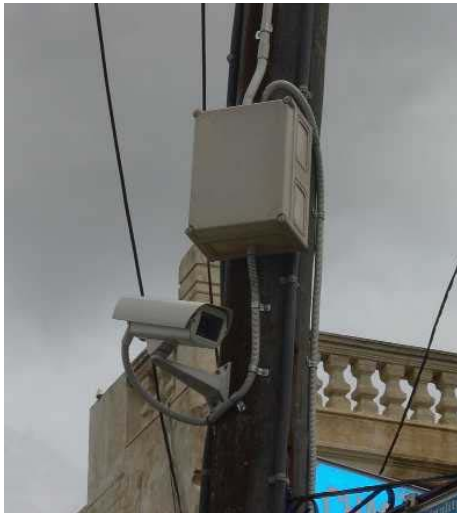
Figure 11: Typical CCT installation
