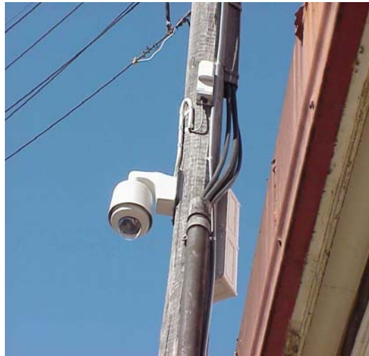
Figure 12: Typical wireless camera installation with mini panel antenna mounted above
