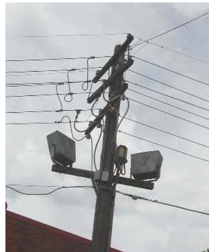
Figure 10: Pair of security flood lights mounted on a separate cross arm
