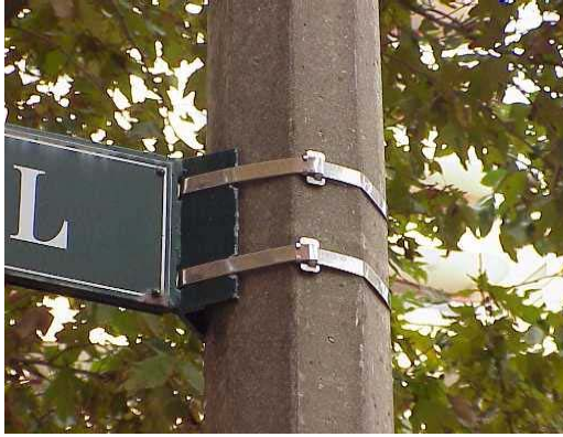
Figure 21: Road sign secured to a concrete column with stainless steel band clamps
