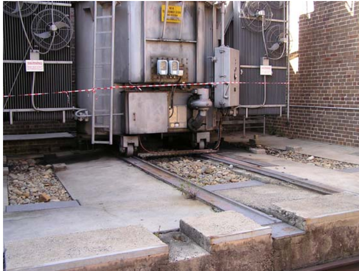
Figure 2: Oil Containment Bund with Gravel
