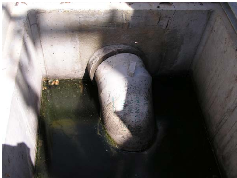
Figure 6: Typical Flame Trap (grate removed for photo)
