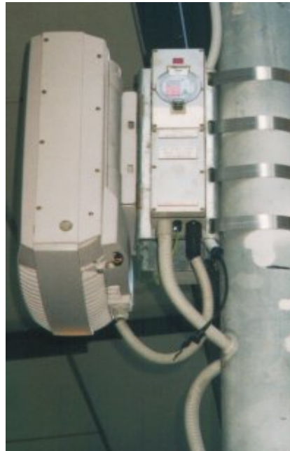
Figure A4: Third Generation Telstra PS on column
