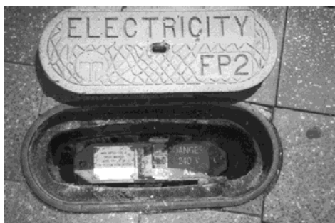
Figure 3 Telstra Electricity Pit
