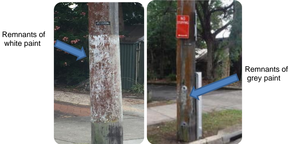
Figure 1: Examples of poles with remnant friable asbestos containing paint
