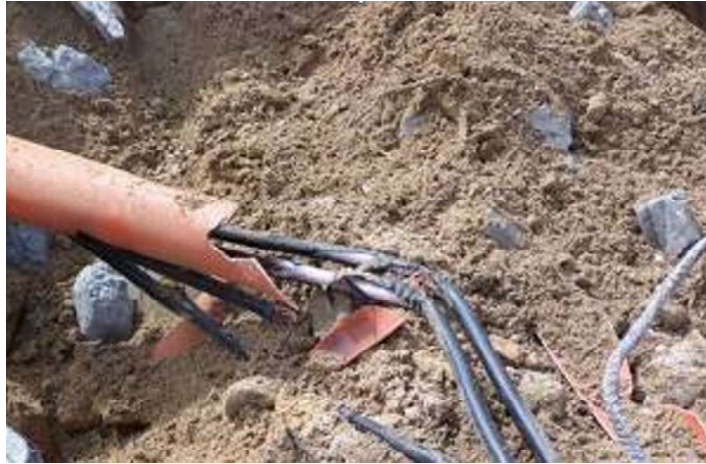
Figure 8: Example of damaged Ausgrid asset
